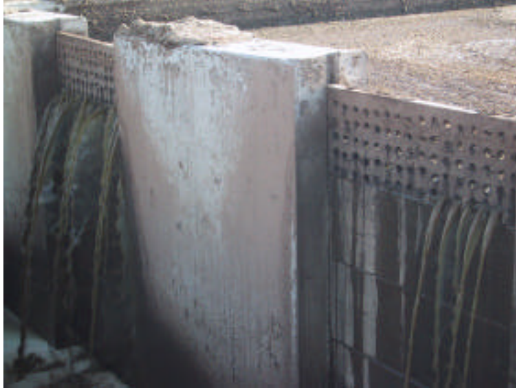
Weeping Wall with Clogged Holes
